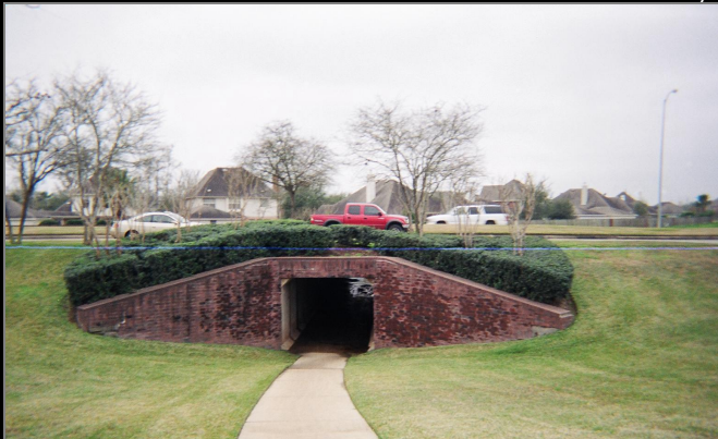
Pedestrian tunnels and other improvements are necessary to overcome barriers to pedestrian mobility.
